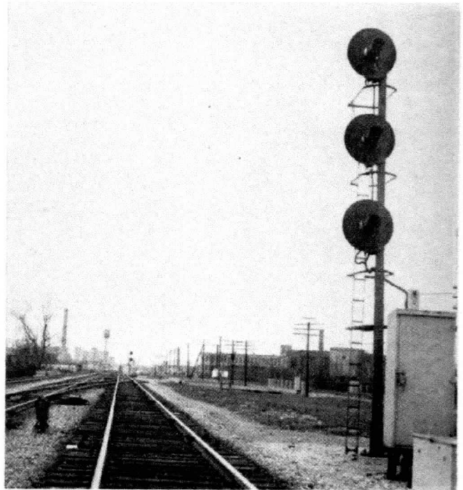
View of signals 22L and 16L looking toward West Detroit
